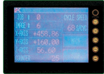
PLC control with touch screen interface
